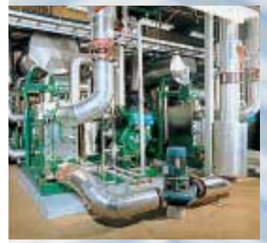
The AlfaRex TM10-B ammonia evaporator and condenser in a chiller heat pump system with ammonia as refrigerant installed in a Danish research institute. The system was built by Sabroe.
