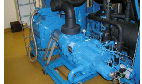
Ethyleneglycol Chiller Unit
